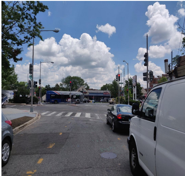
Poor pavement markings on Kalmia Road, NW
