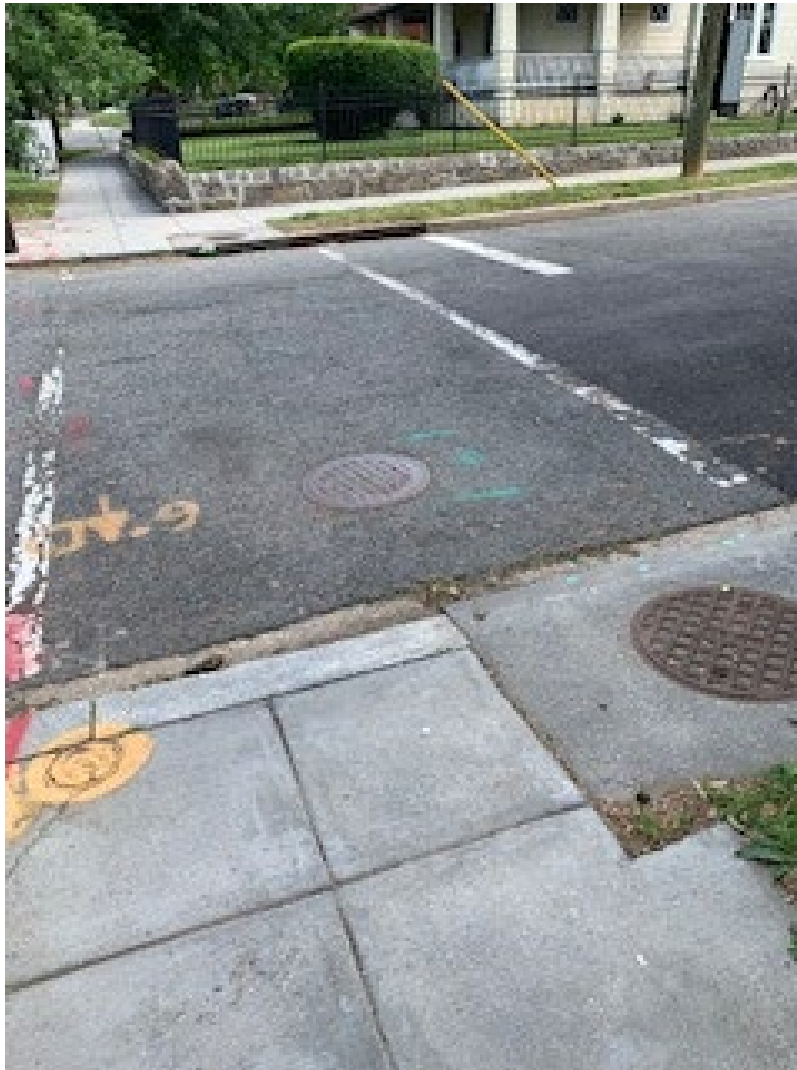
Figure 4: Missing Curb/ADA Ramps on the East Leg of the North Capitol Street and Kennedy Street NE Intersection
